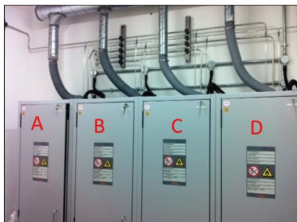
Figure 2: SFC co-solvent delivery room and flammable solvent cabinets for each solvent type methanol (A), ethanol (B), isopropanol (C) and special solvent blend as required (D).
